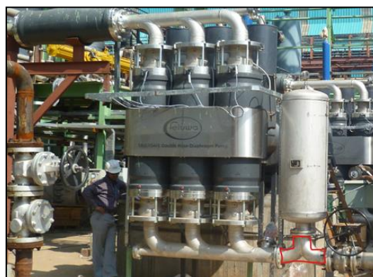
Figure 4. The bottom short piece of the suction accumulator (highlighted) of the double hose-diaphragm pump at the autoclave area of UCIL, Tummalapalle Mill
