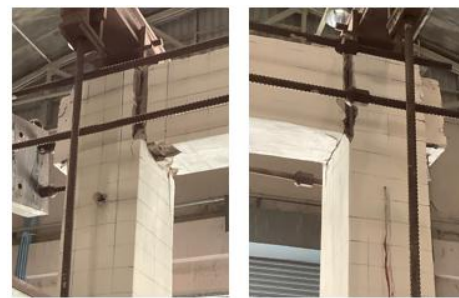
(b) Cracks of the beam-column joint
