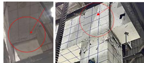
(b) Cracks at the upper of beam-column joint
