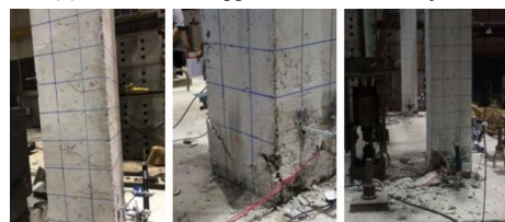
(c) Cracks at the upper of beam-column joint
