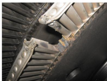
Figure 1 The Fracture at the root of the 5 th rotor wheel's blade. Adapted from “Steam turbine moving blade failure caused by corrosion fatigue - case history” by Katinić, & Kozak (2018).
